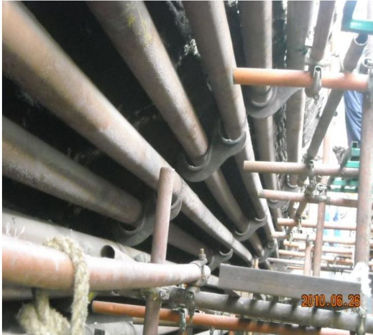
Vacuum Section horizontal tubes
