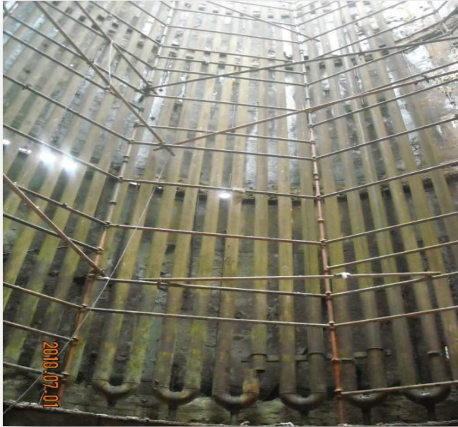
View showing Vertical Heater Tubes arrangement.
